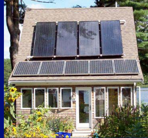
Hot Water Panels
