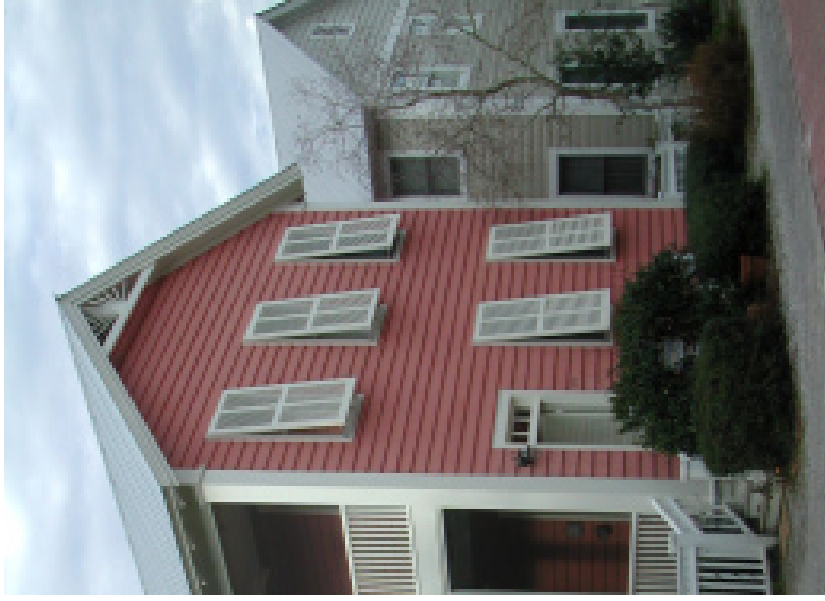
Where is the A.C. condenser?
