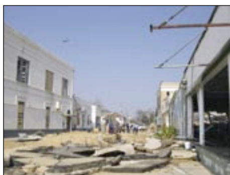
VIEW OF THE DAMAGE TO THE BUILDINGS ON MAIN STREET IN BAY ST. LOUIS
