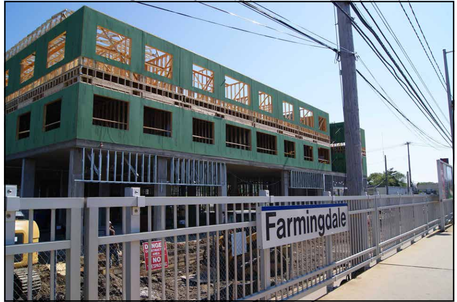
Jefferson Plaza, a transit-oriented development at Farmingdale Station on the Long Island Rail Road. Photo courtesy of Vision Long Island.
